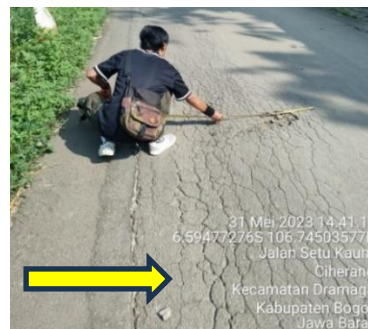
Figure 6. Crocodile Crack 0+500 - 0+600. Source: Research data
