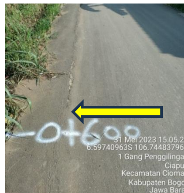
Figure 7. Longitudinal crack 0+600 - 0+700. Source: Research data
