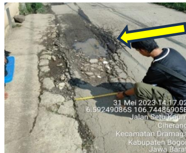
Figure 4. Pavement Edge Defects at Sta 0+100. Source: Research data
