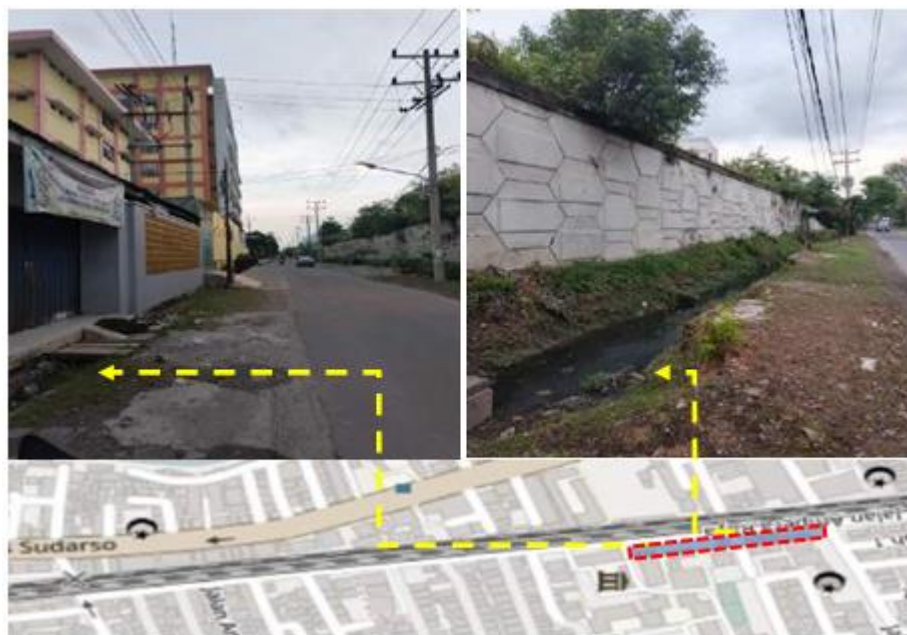
Figure 8. Existing Condition of the Ampera Road Drainage Network in Medan Analysis of the Drainage Network System in Ampera Road in Medan
