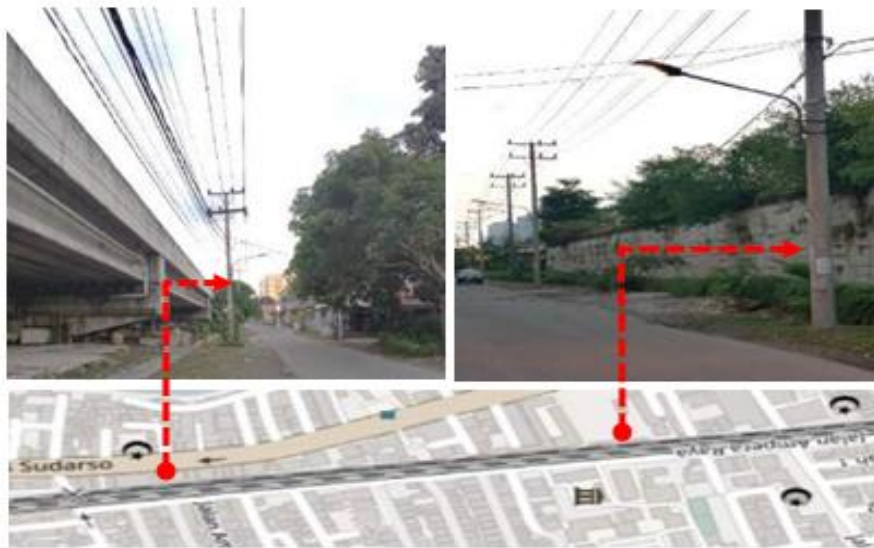
Figure 4. Utility pole equipment in the Jalan Ampera Medan corridor
