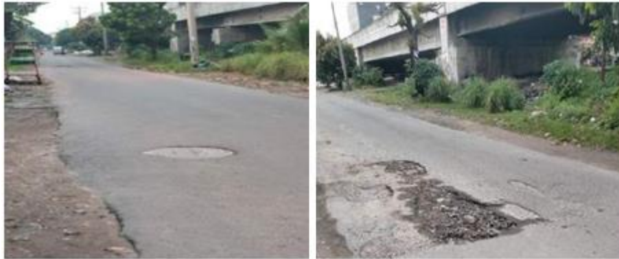
Figure 2. Road damage due to Ampera road utility work
