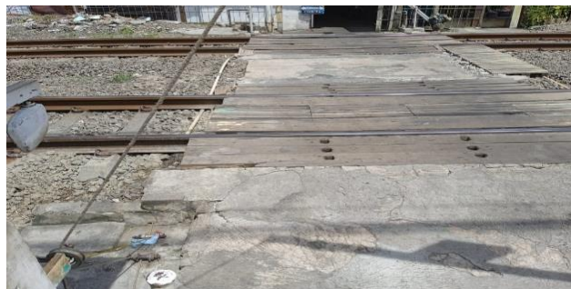
Figure 2. Illegal Railway Level Crossing Source: Personal Documentation
