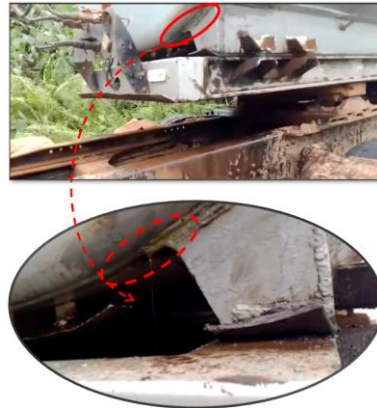
Figure 6. Details of the Leak on the Bottom of the Front of the Tank
