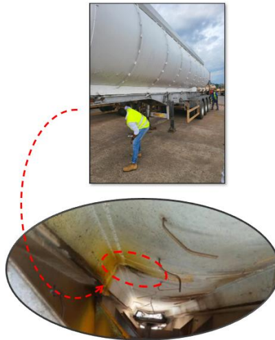
Figure 4. Details of Leaks on the Lower Side of the Middle of the Tank
