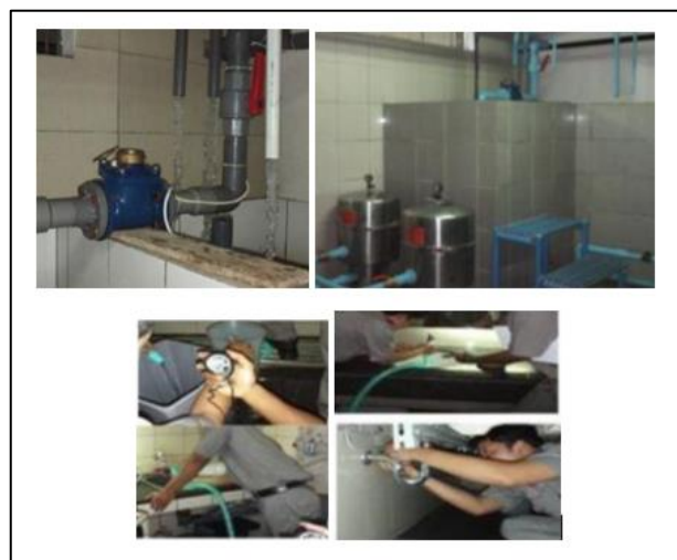
Figure 3. Rainwater Treatment, Seepage and AC Condensate
