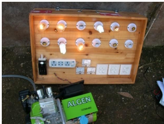
Figure 6. The cross-section of the observation of the generator loading
