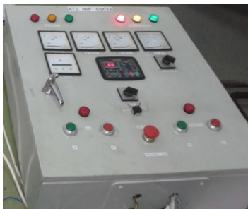
Gambar 6 Panel ATS/AMF 66 kVA, 380 V, 50 Hz
